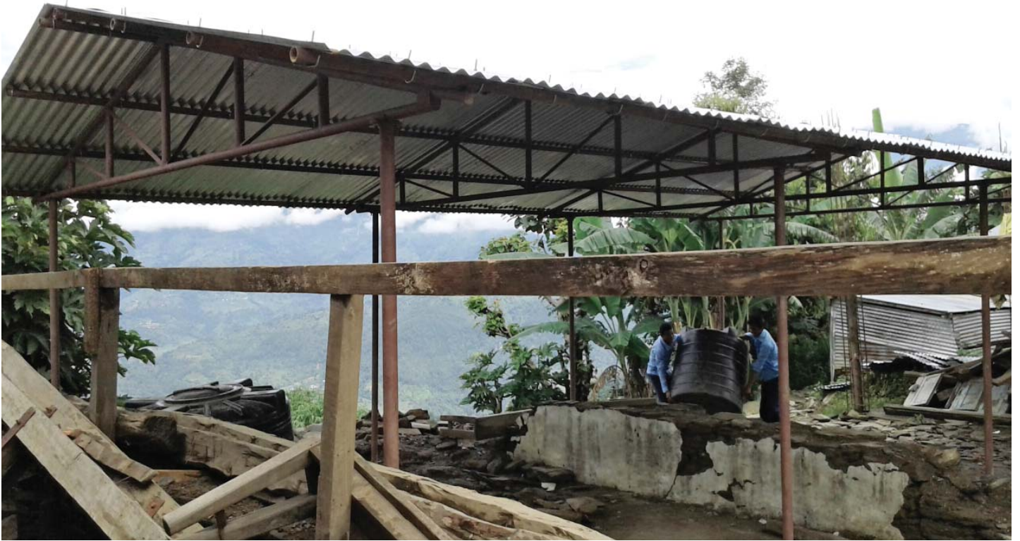
Photo (top): one of the trusses commissioned by us installed at the school over one of the previous classrooms (thanks to the school for providing the photo)
