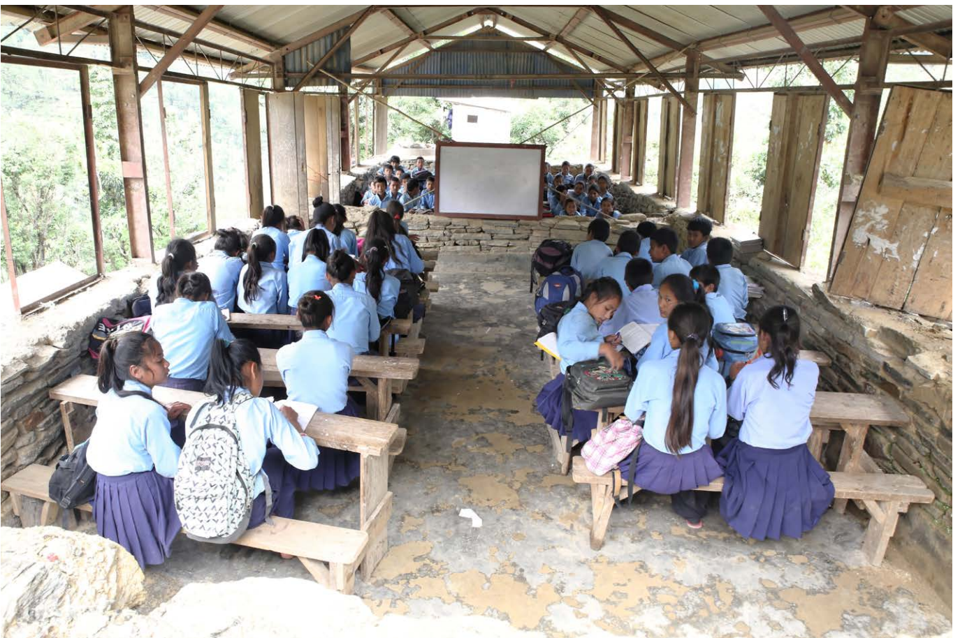
The photos above are of the existing Nabin School buildings that were seriously damaged and condemned during the government survey of schools in the earthquake zones. So teaching could resume quickly, the walls were removed to make them 'safer' should another tremor strike. In the bottom photo, the fact that two classrooms with no walls are facing each other makes it difficult to conduct classes. Not all the rooms had their walls demolished, the top photo showing grade one children in a room where the rear wall collapsed but the rest of the building remained relatively intact.
